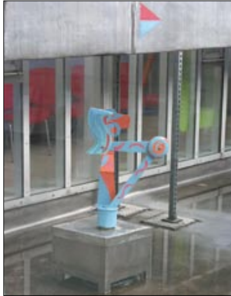
Commissioned sculpture adds interest to external pipework (right)
