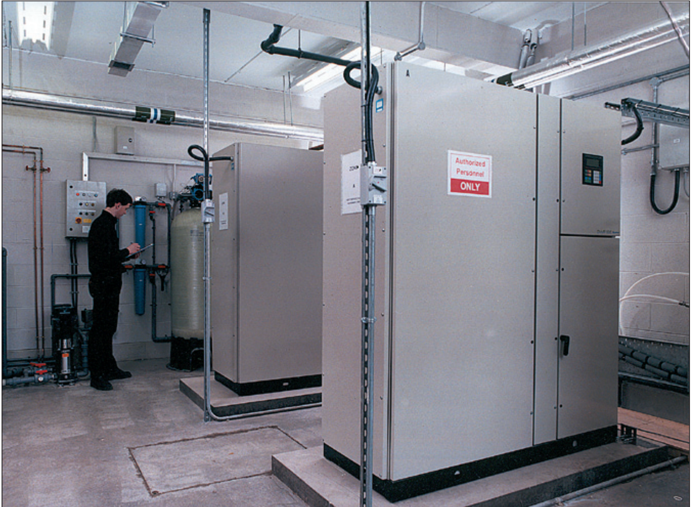
The quality of water that can be achieved with a central water-treatment plant is generally far higher than that which can be obtained from individual units. Courtesy of Esler Crawford Photography; reproduced by kind permission of Belfast City Hospitals Trust
