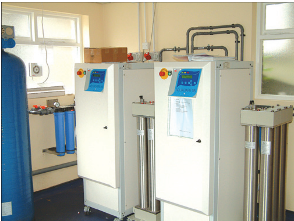
Water to be used for dialysis needs to be treated appropriately to remove impurities. For normal haemodialysis, water purity must meet the minimum standards for regular water quoted by the European Pharmacopoeia
