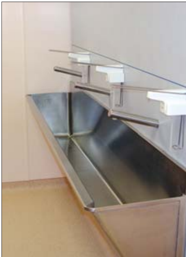
Figure 8 Scrub sink with non-touch taps
