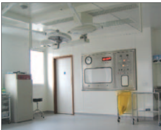
Figure 10 Theatre control panel
